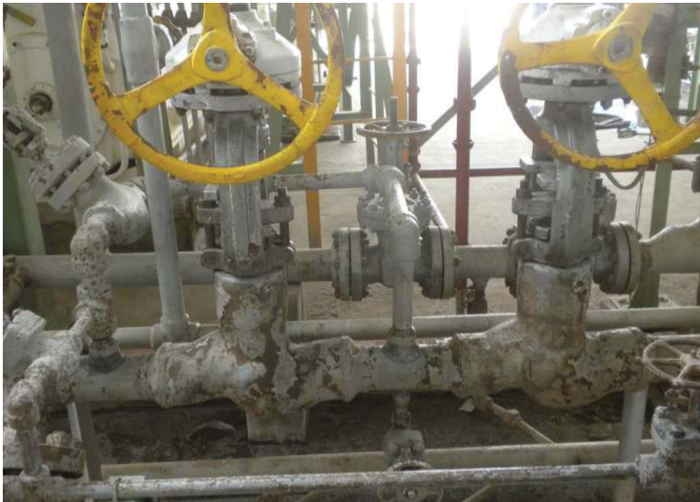
Damaged painting & atmospheric corrosion observed on NH-9002
