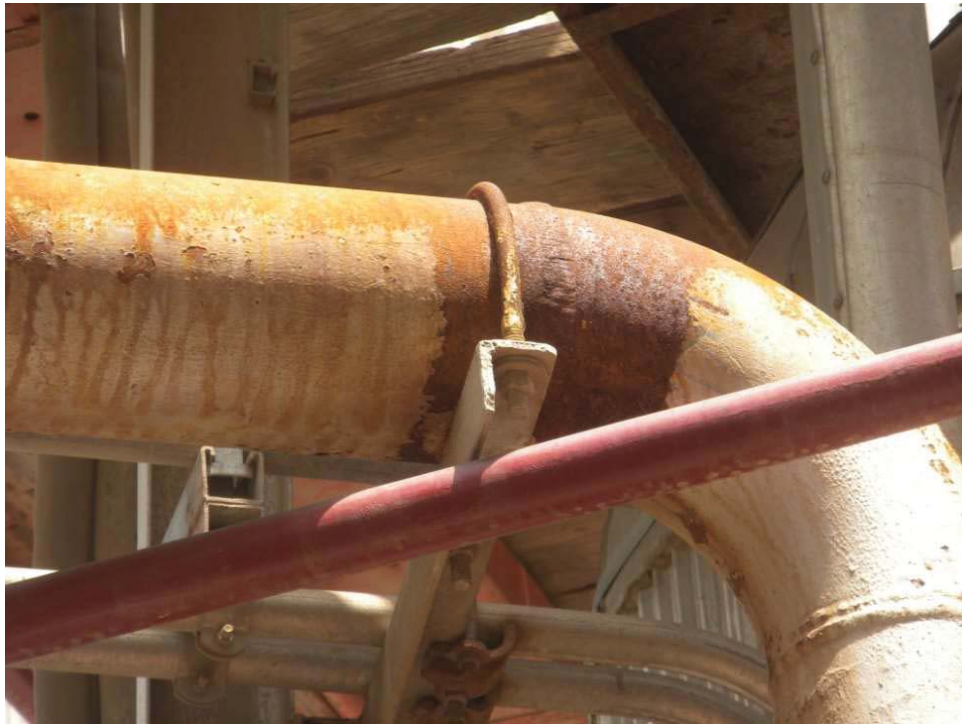
Preferential atmospheric corrosion observed at support locations of CO-9005
