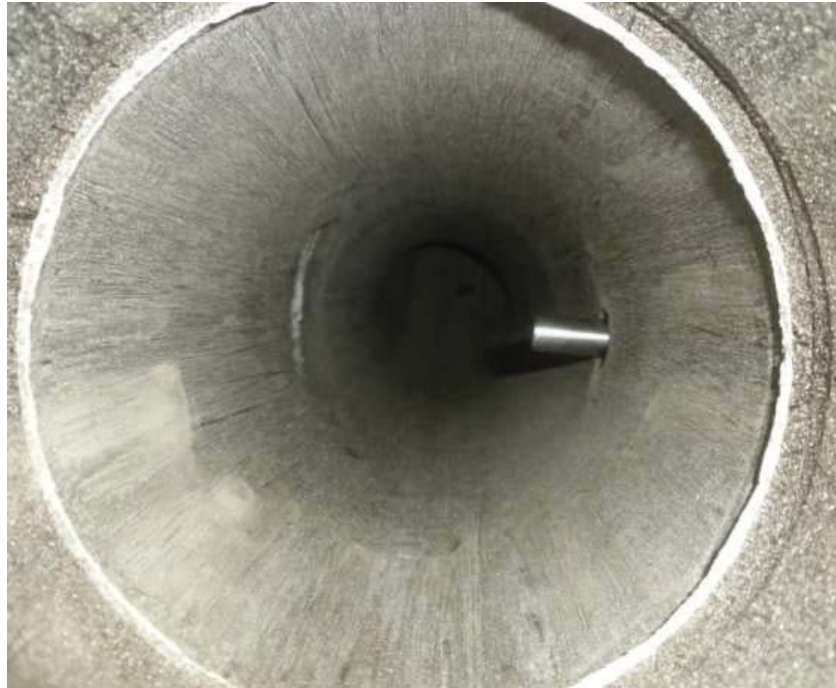
Uniform Corrosion observed in CB-9005 & other liquid lines
