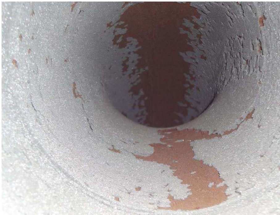
Condensation Corrosion observed in Wet Gas Lines
