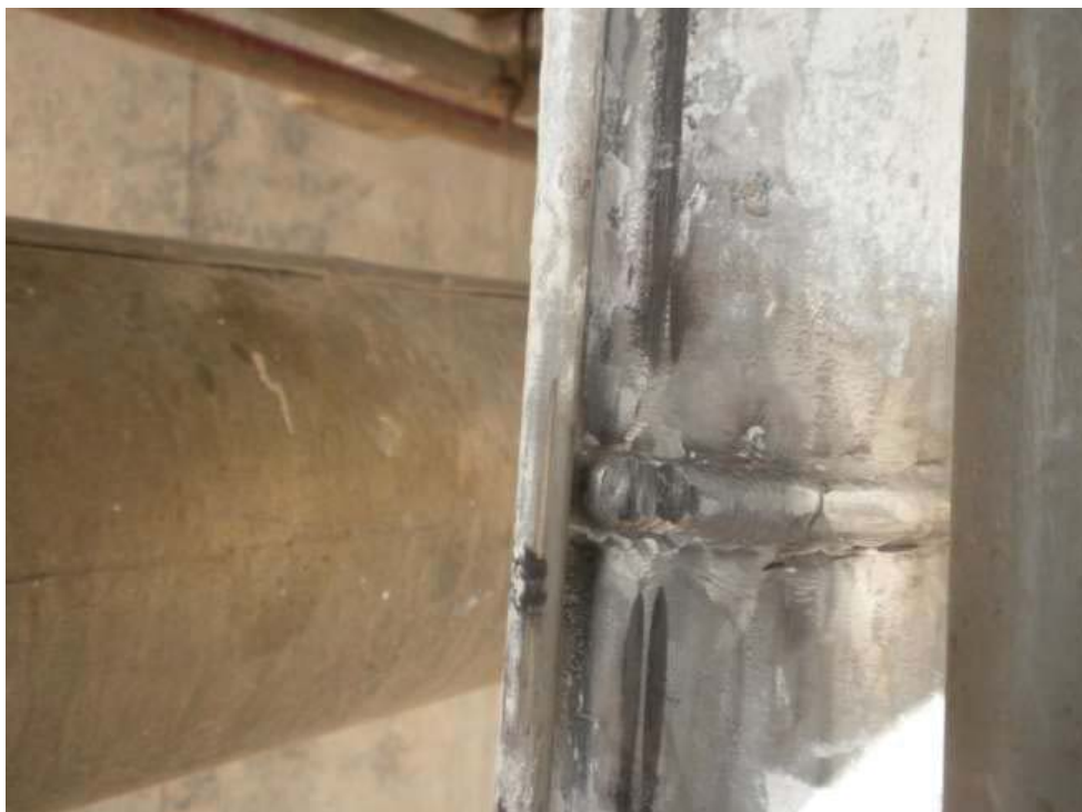
Mechanical damage (rubbing) observed on CB-9007 between Platforms 4 & 5
