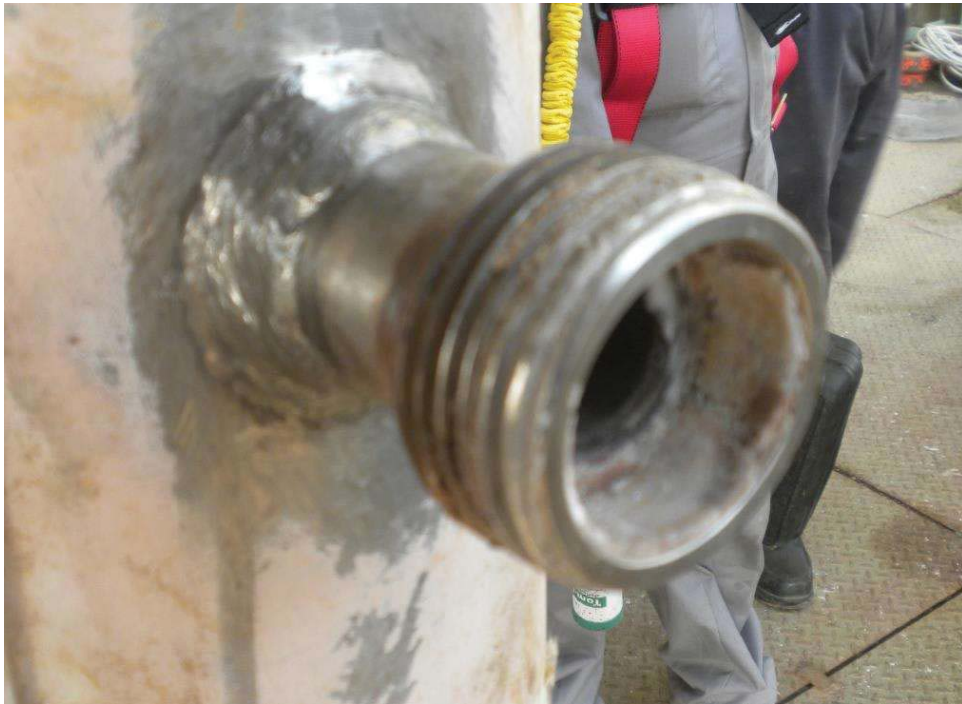
TE-9051 weld-o-let found severely corroded from inside
