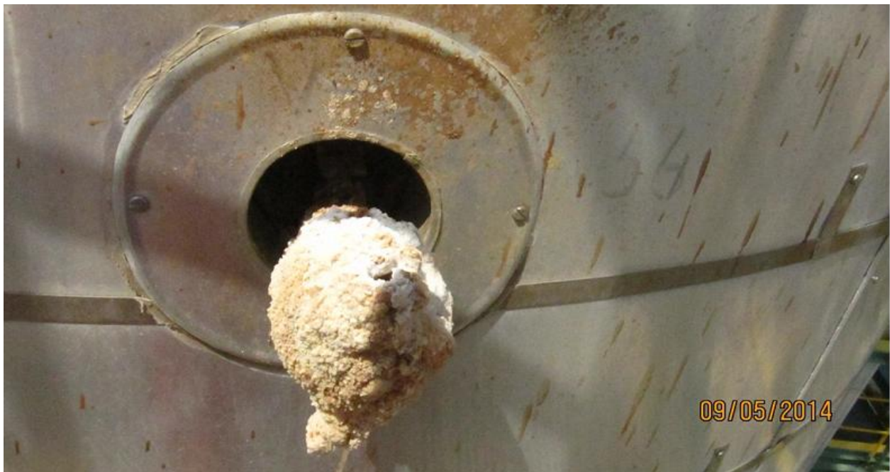
Fig. 3: (Leakage through Weep hole)
